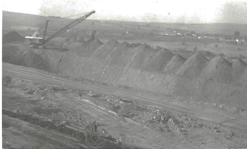
In the above photo a trench is being excavated by a large dragline and the debris piled onto a
